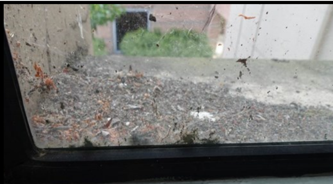
Window ledges throughout the second floor have accumulated dirt, debris and bird droppings.
